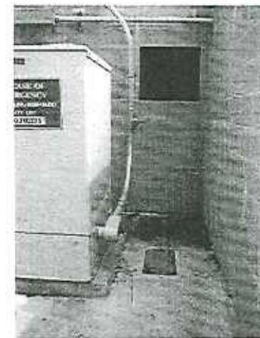
NEW FIBER EQUIPMENT LOCATION
